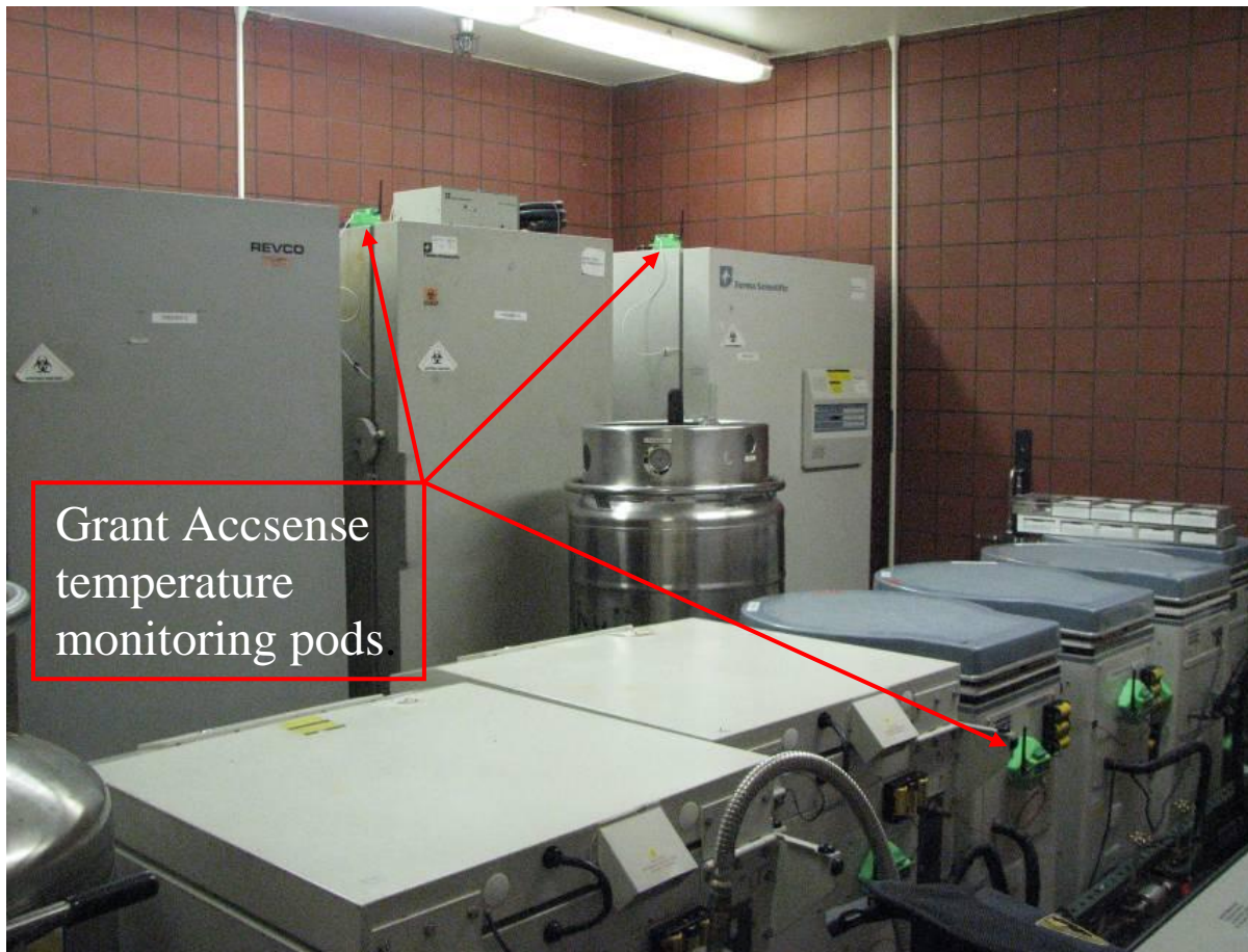
A 35-unit cryogenic installation at a major University Research Center, showing both LN 2 and mechanical freezers.
