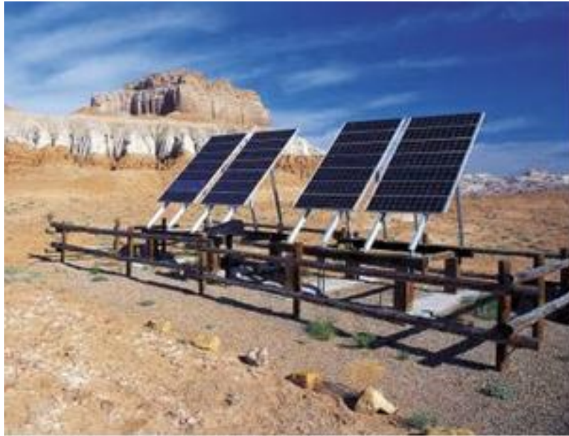
Remote solar facility.
